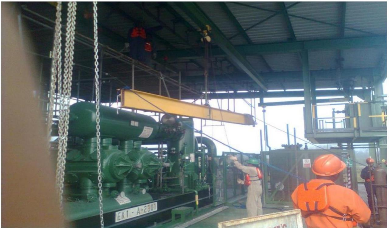
MANUAL LIFTING OF BEAM FOR INSTALLATION AT EKULEMA AGG INSTALLATION OF OVER HEAD CRANE AT EKULEMA AGG BY OGFYG .CLIENT SPDC
