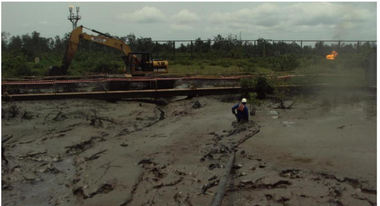
RIVER CROSSING FOR PIPELINE LAYING WITH SWAMP BUGGY AT AWOBA W3L BY OGFYG Nig.Ltd. CLIENT SPDC RIVER CROSSING FOR PIPELINE LAYING WITH SWAMP BUGGY AT AWOBA
